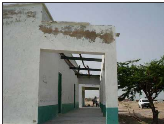
Figure 4: Blew away roof top of a building in Chandi Village. Photo credit: Ahmad Khan
